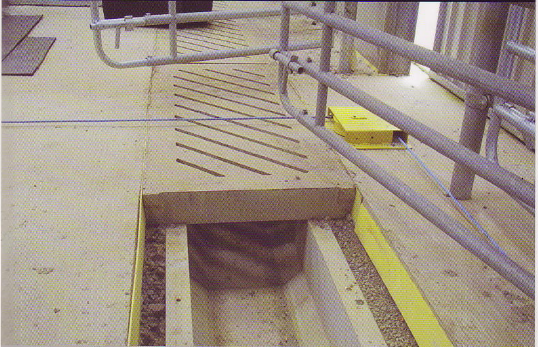
Slurry channel systems
